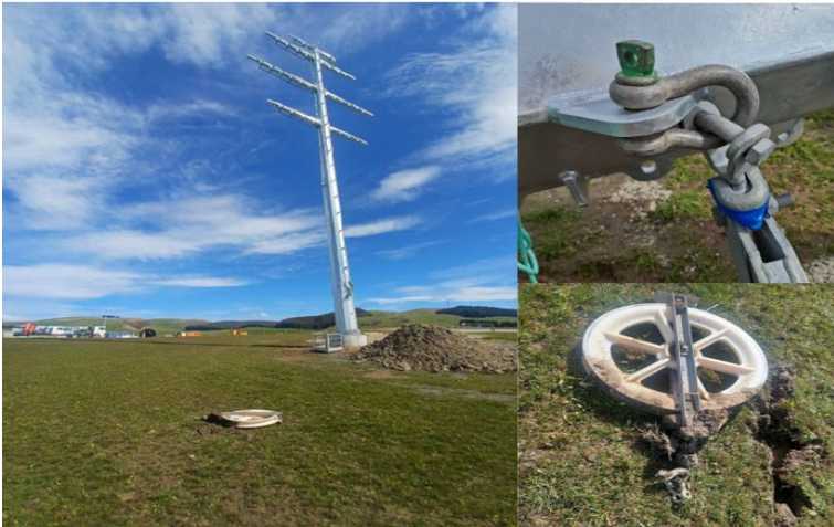
Figure 1. Distance from the pole to the ground where the running block had fallen. Shackle used without a secondary restraint.
